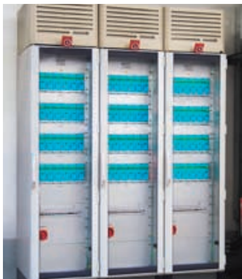
The SONIC-digital generator series in the 19-inch version of the air conditioned control cabinet
